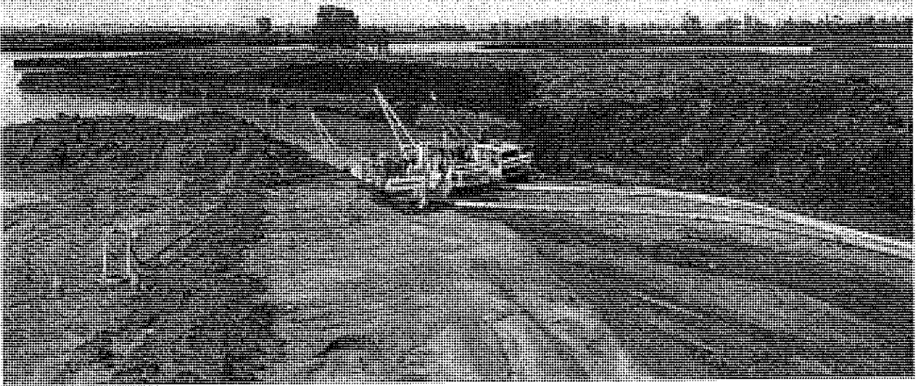
Typical Bunded Pump Fuel Tank Installation (currently Ramp 26 East)
