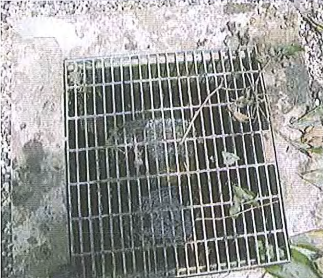
14/01/2011, 1:04:34 pm: Stormwater grate beside Aura property showing where water bubbled up and forced the mud aside
