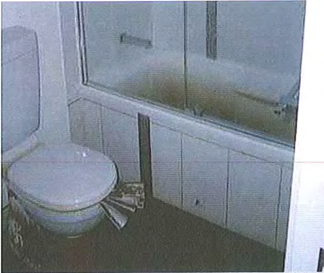
13/01/2011, 4:00:02 pm: Toilet and bath (Unit 4, ground floor of Aura) showing muddy water that came up through plumbing
