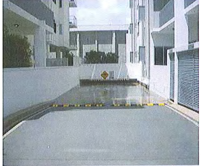
12/01/2011, 10:29:00 am: Entrance to Aura's basement showing water filling the basement but no water going over the lip as yet
