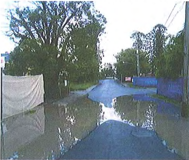
12/01/2011, 5:21:59 am: Ferry Road looking towards the river showing stormwater in Ferry Road
