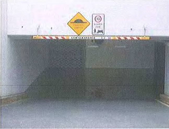
12/01/2011, 7:47:42 am: Showing a dry driveway at the entrance to Aura's basement 1 with water pooling at the bottom
