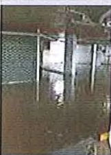
12/02/2011, 3-4.00 am: Entrance to Aura Basement 1 showing water coming in vents
