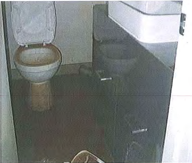
14/01/2011, 12:10:13 pm: Aura common room toilet with flood line on pedestal & muddy waters overtopping bowel from inside
