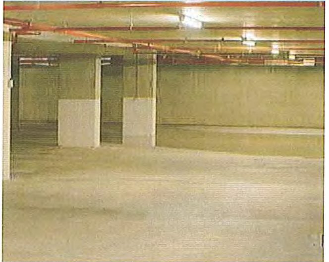
12/01/2011, 1:20:24 am: Water beginning to spill across floor in Arriva basement carpark
