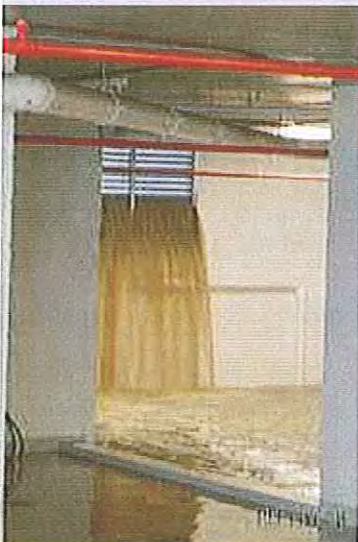
12/01/2011, 7:15:48 am: Water spilling through vents into Basement 1 in Aura
