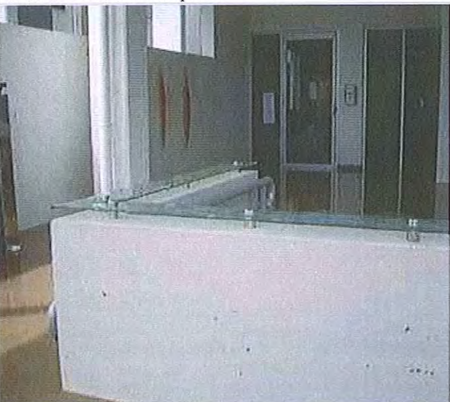
13/01/2011, 10:01:05 am: Water pooling in the entrance to Aura Apartments
