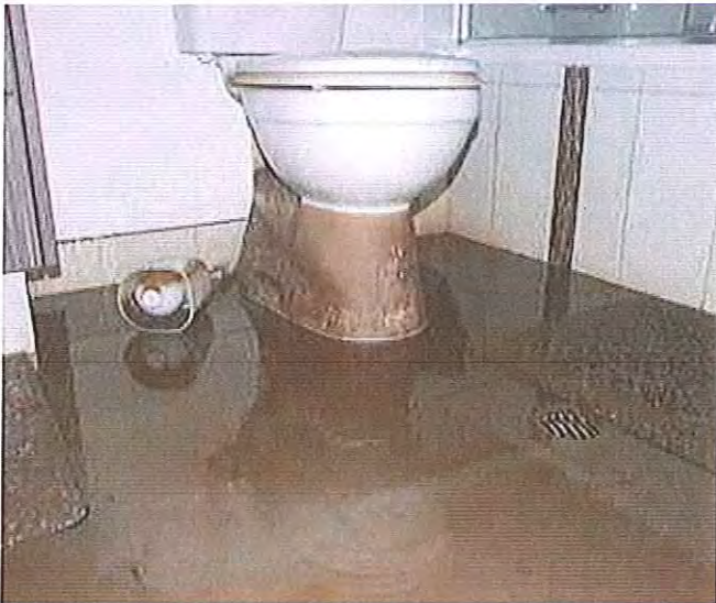
13/01/2011, 10:05:48 am: Ground floor unit toilet showing the level where water came up through the drain hole in floor
