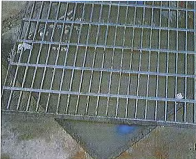
12/01/2011, 1:20:02 am: Grate above submersible pumps in basement of Arriva Apartments next door to Aura
