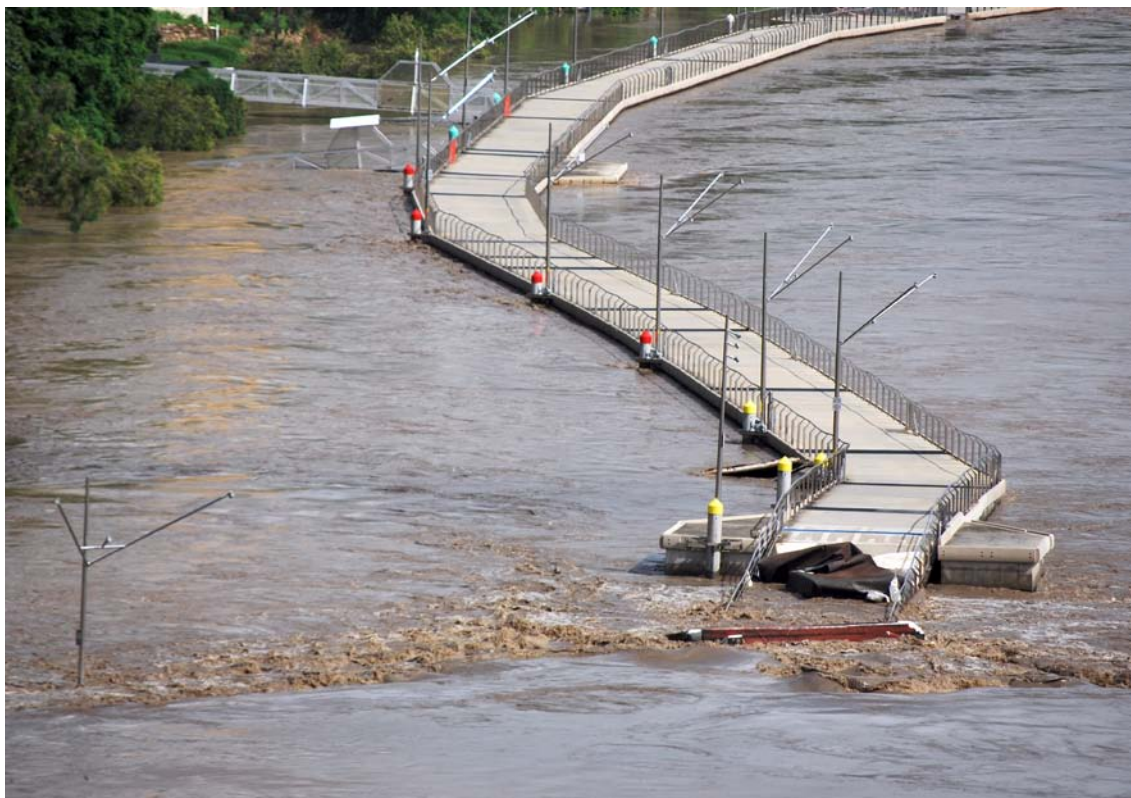
Flood damage to New Farm Riverwalk (photo courtesy Stephen Knight)
