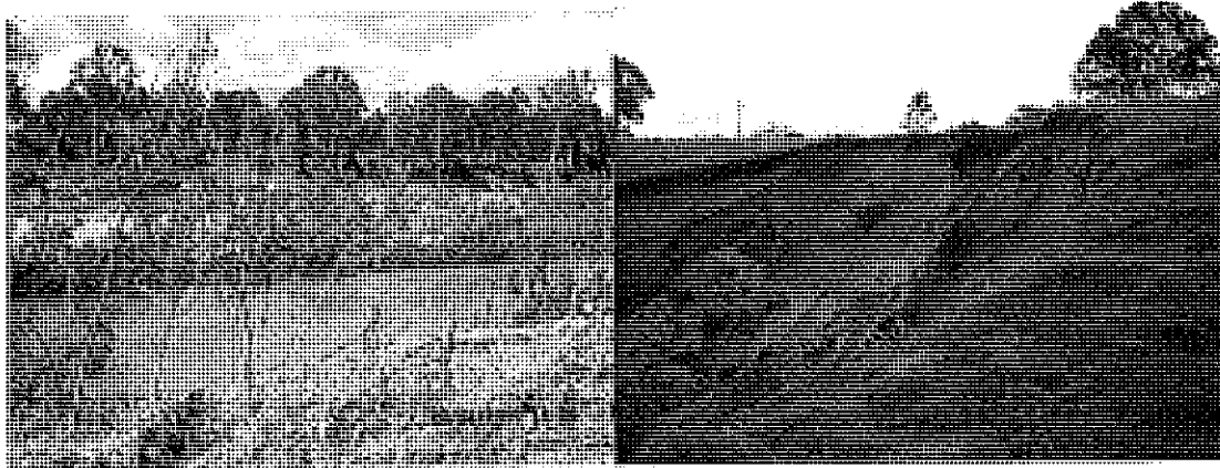
Massive scarring on Lowood – Fernvale section
