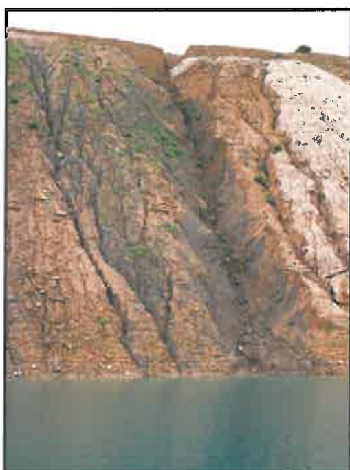
Figure A1.7: Large eroded gully in spoil
