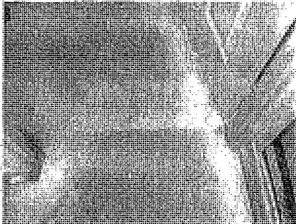
Photo 7: Slab cracking at Robe Entry
