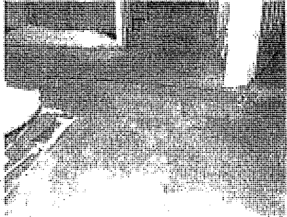
Photo 8: Slab distortion at Bathroom
