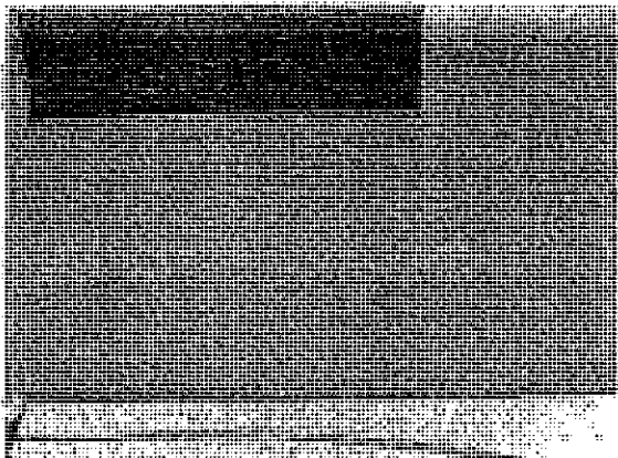
Photo 15: Cracking in Panel at Window
