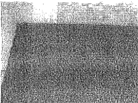
Photo 17: Minor crack in Plaster
