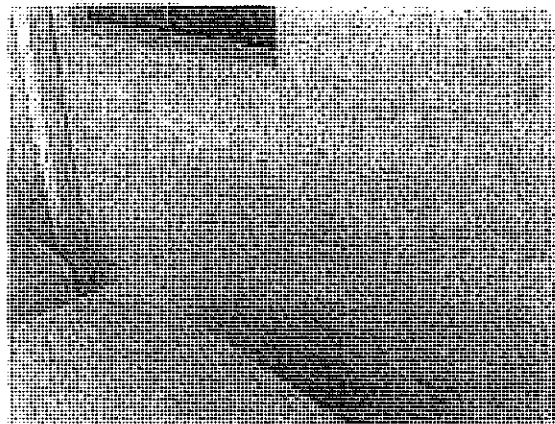
Photo 14: Cracking in Panel at Window
