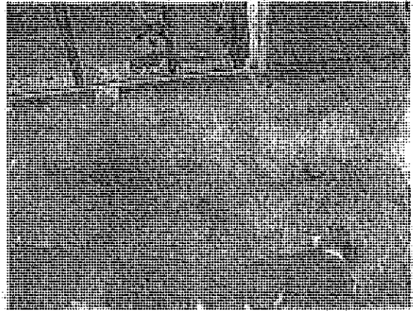
Photo 2: Slab cracking in Bedroom 3
