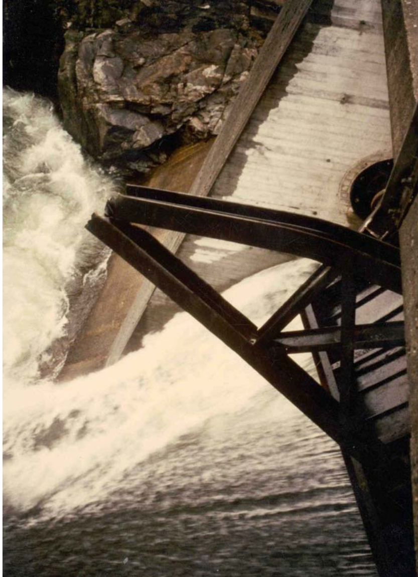
Photo 7 Gate Failure: Ulefoss, Norway Photo Supplied by H. Fosker of Norconsult, Norway
