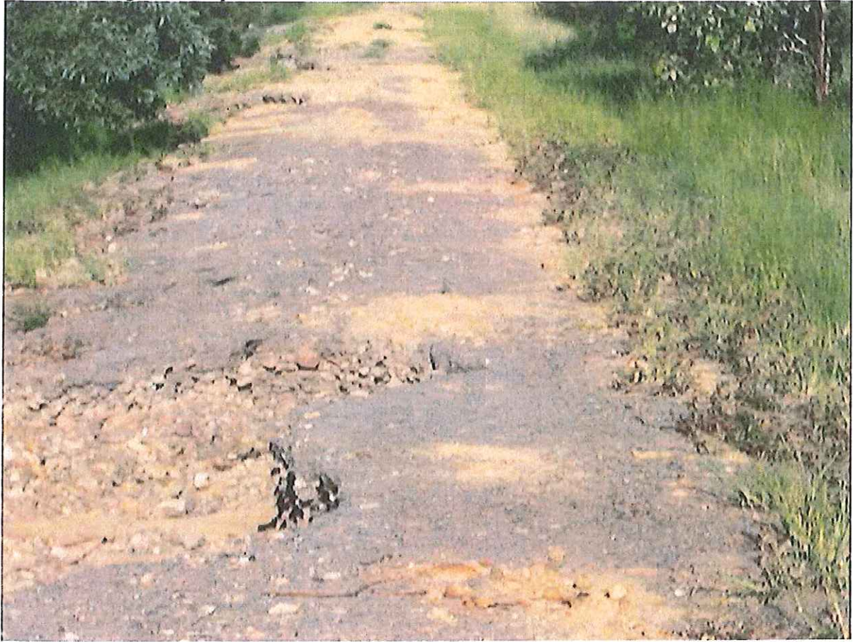
View of damage at other points of Rail Trail
