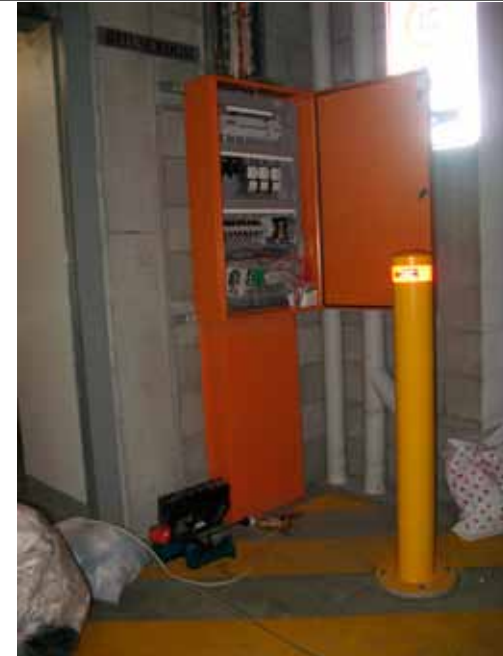
CO 2 Panel controls in Basement 1 beside the lift shaft
