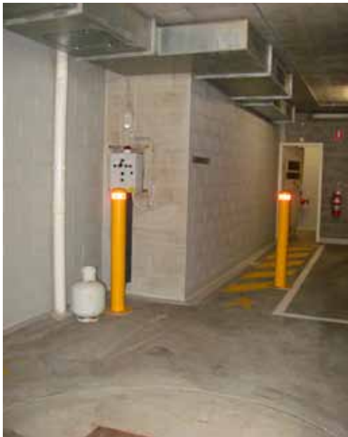
De-watering pump controls in Basement 2
