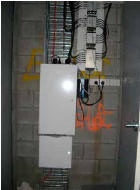
Video cabling controls located on ground floor
