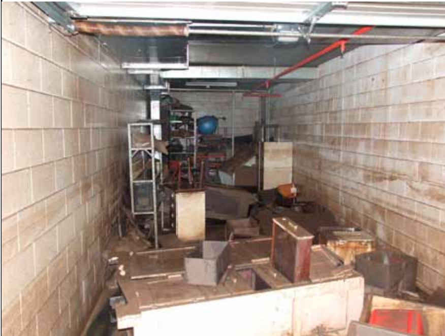
Metal ducts in the roof are part of the CO2 ventilation system
