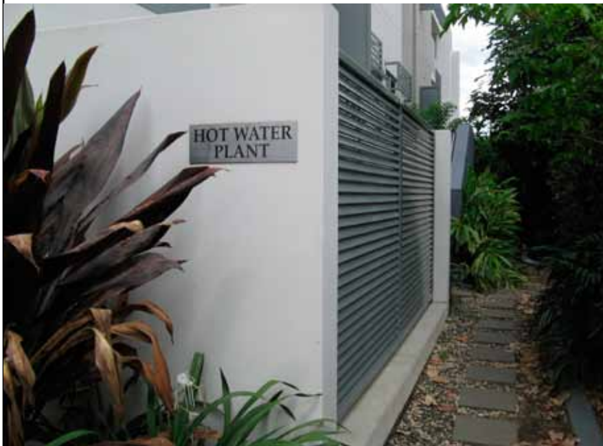
Room housing the water heaters beside the building and well below the building ground floor
