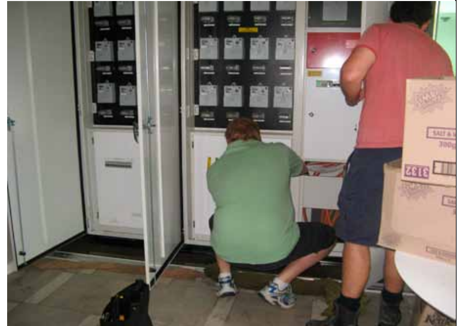
The main isolator switch on the power board was located at the lowest point on the panel and was the most expensive power component to replace
