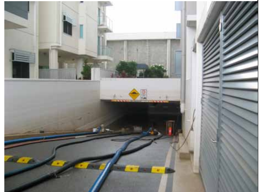
Carpark entrance with a mud line showing the height of the water
