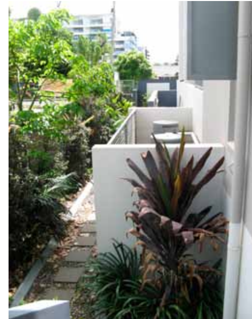
Looking down on the water heaters from the entrance to the fire stairs at ground floor level
