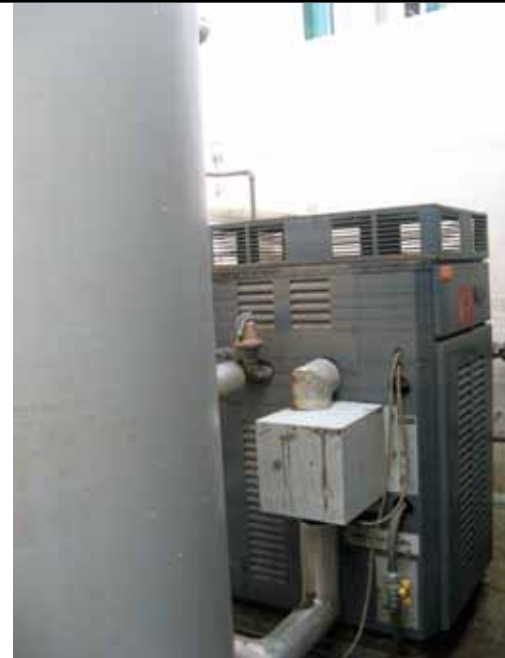
Water heater controls that were completely submerged and damaged by water
