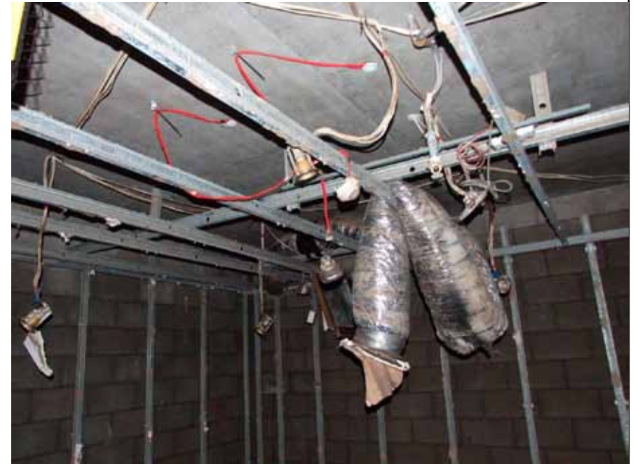
Part of the CO2 ventilation system
