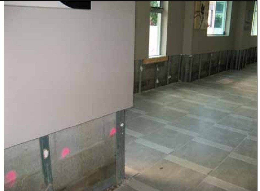
Damaged walls in the Aura foyer
