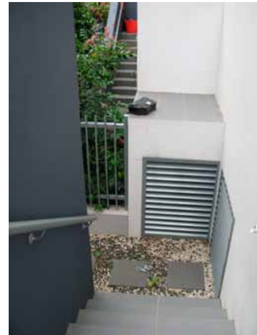
Stairs from ground floor leading to back garden with vents where water spilled into B1 carpark
