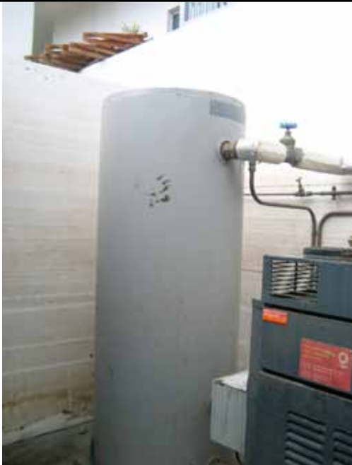
Water heaters that were completely submerged and damaged beyond repair
