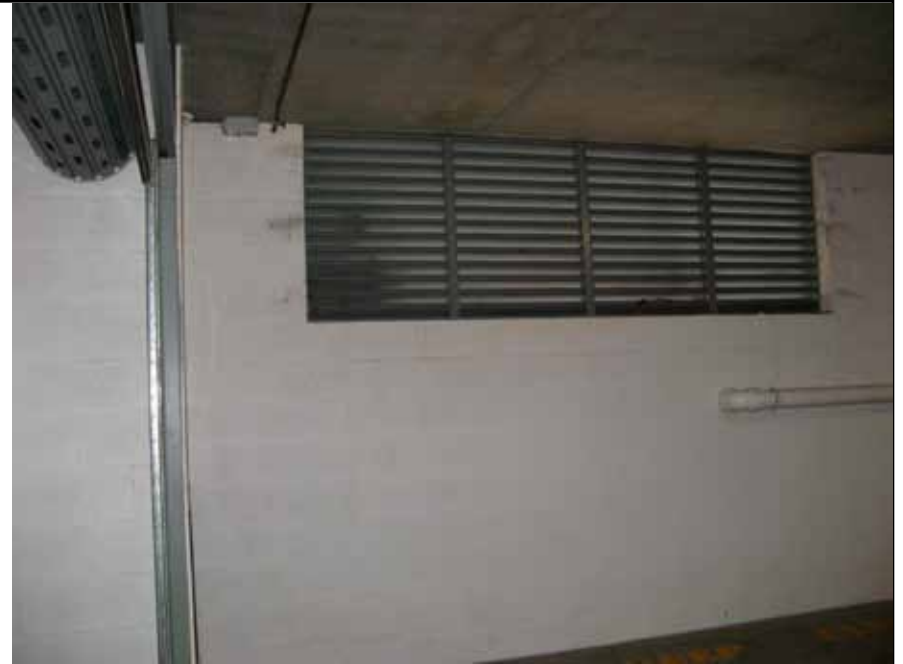
Basement 1 vents where water entered carpark
