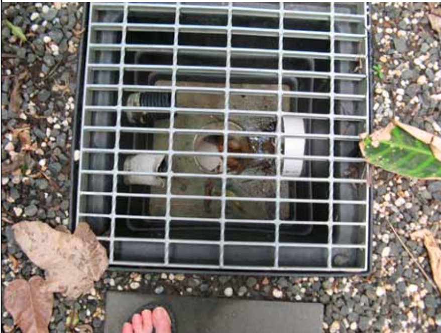
One of smaller grates giving access to the stormwater drain around Aura
