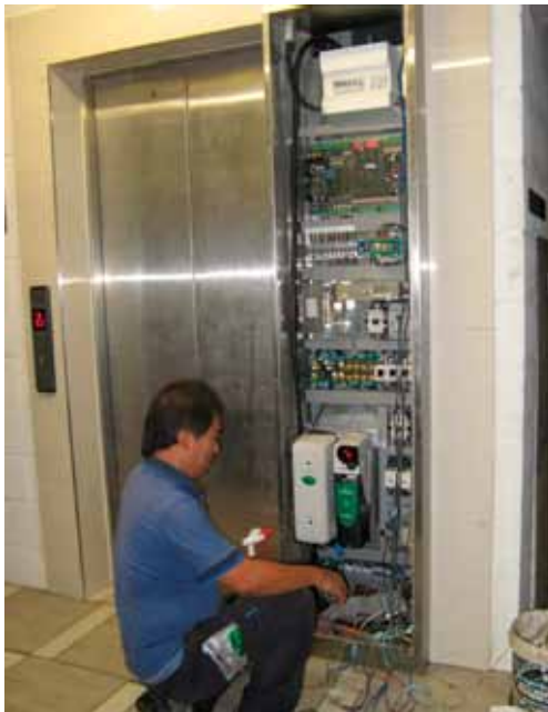
Aura lift control panel beside the lift in Basement 2 positioned at the lowest point in the building
