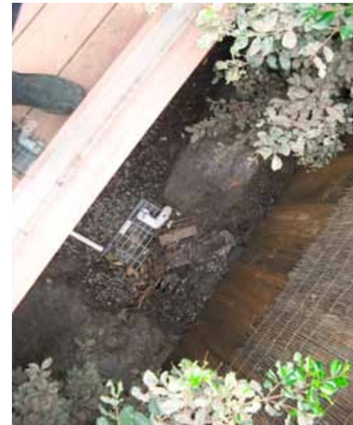
Aura stormwater drain on 14/01/11 at 2.53 pm showing where water bubbling up has not allowed any mud to settle around the grate
