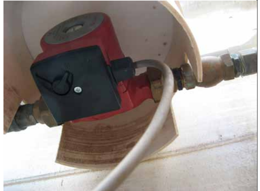
Close up of hot water recirculation pump that needed to be replaced
