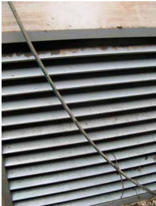
Close up of vents where water spilled into the B1 carpark basement
