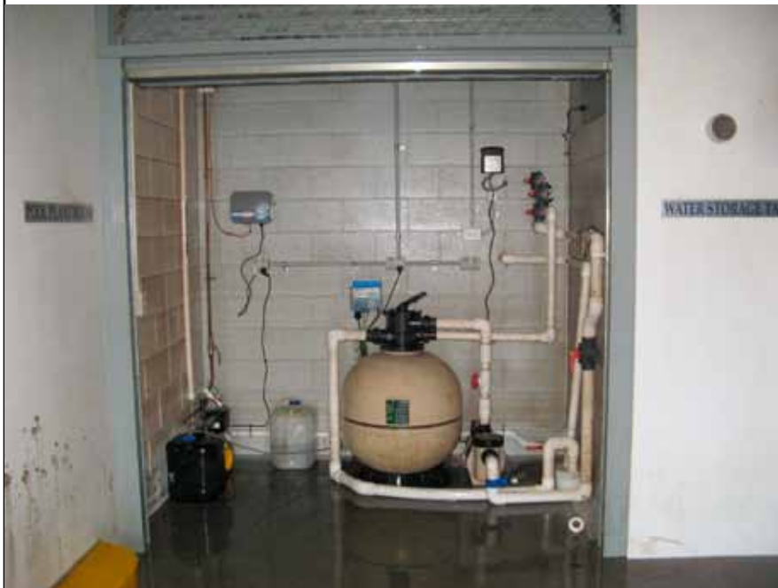
Close up of damaged pool controls in room with door raised on Basement 1
