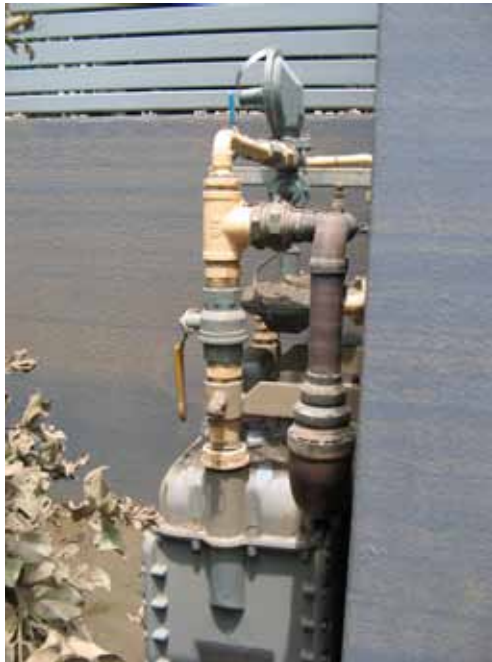
Main gas valve
