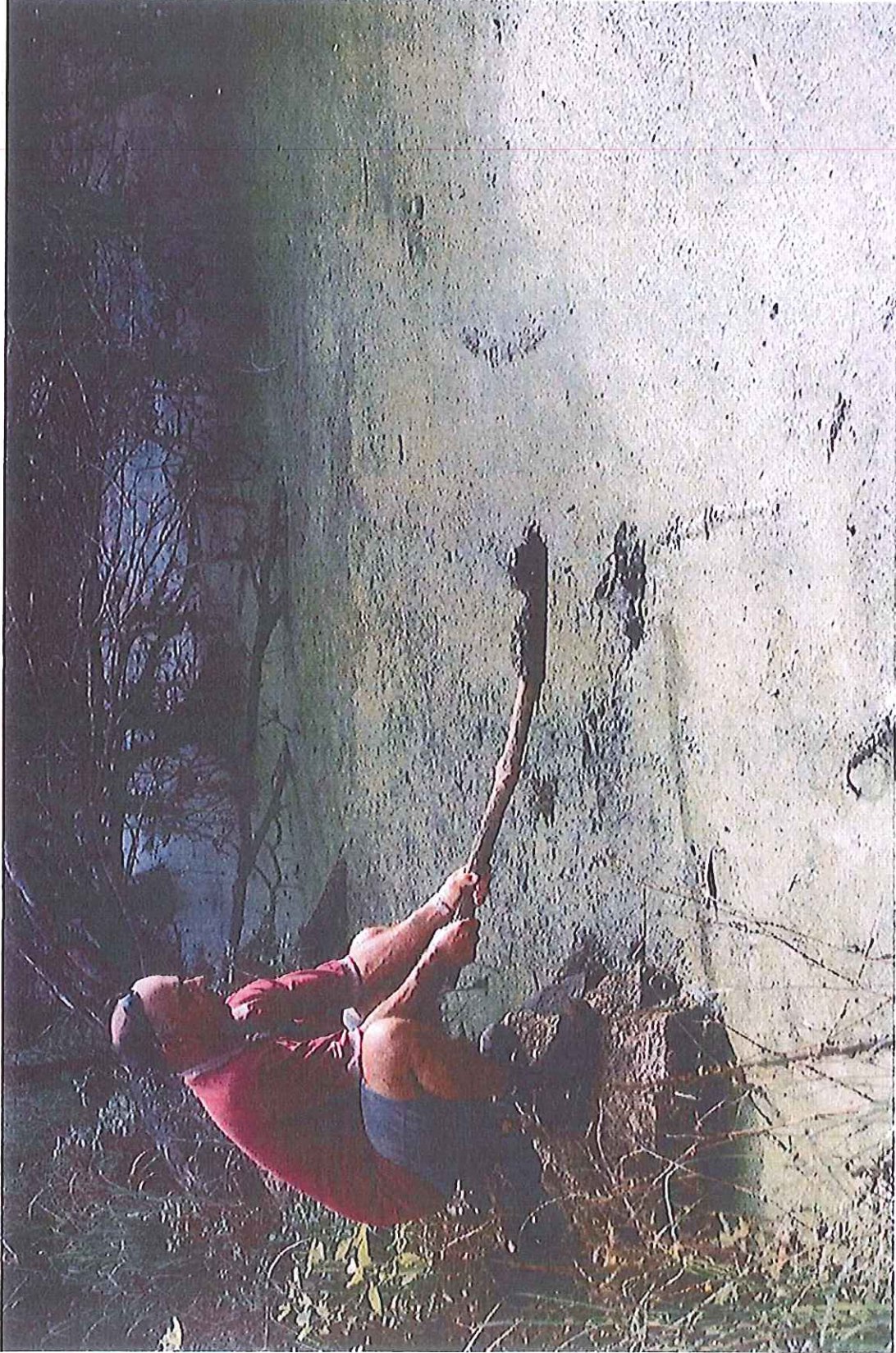
West of tidal wall (outlet pipes 3 x approx 40mm with tidal caps), minimal flow observed, heavy scum on surface for 100m behind.
