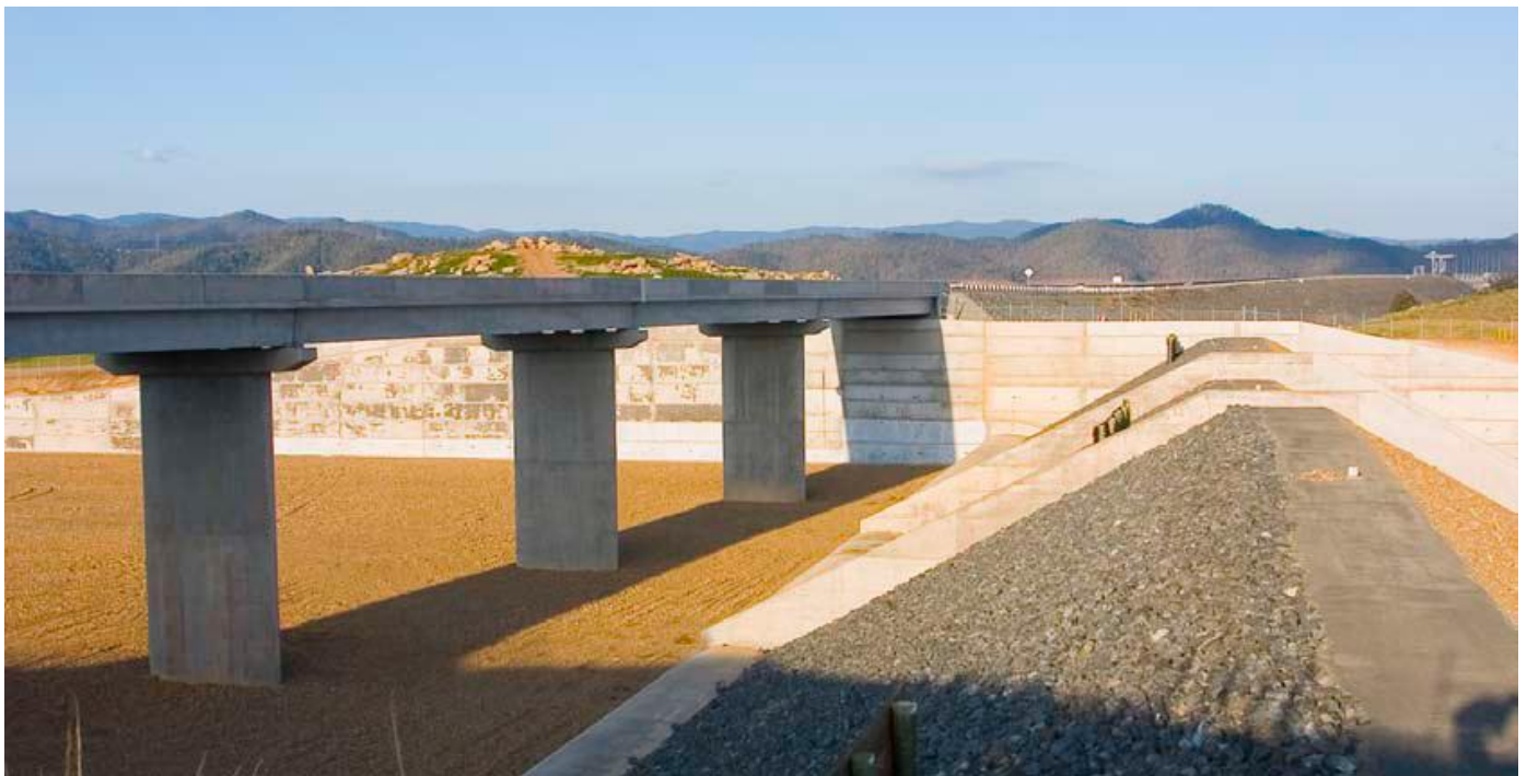
Figure 6: The 3 Wivenhoe Fuse Plugs. Notice the different heights. The Brisbane Valley Highway is at left, the gates at far right.
